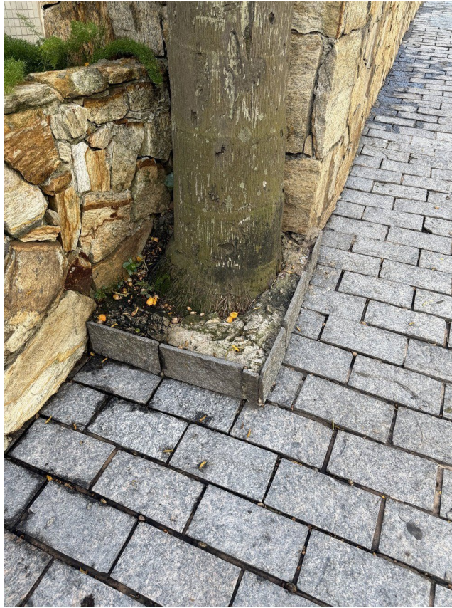
Plate 3. Mature trunk wedged into the linear gap between a stone retaining wall and granite paver field, with effectively no surface pit.
