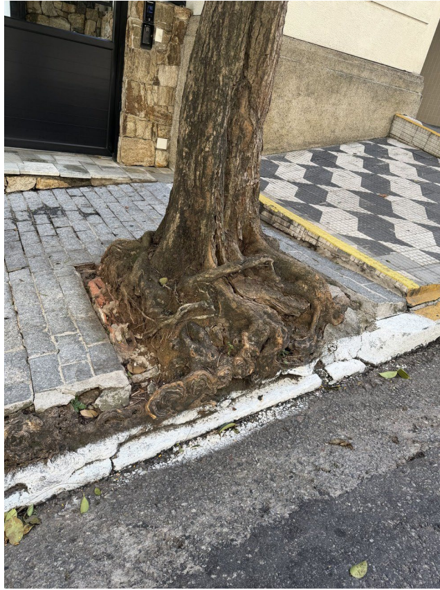
Plate 4. Buttressed root mass overflowing the pit, deflected by the curb edge, with painted curb line distorted by years of incremental displacement.
