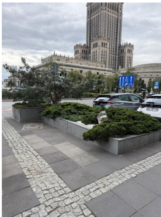
Raised granite planters in the central district: dwarf conifers and prostrate junipers in volume-capped beds. Ornamental hardscape — not urban-forest root-space provision. Note also the visible structural failure in the planter walls.
